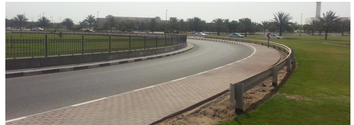
Full height hazard with inadequate anchorage for the guardrail system to perform.
